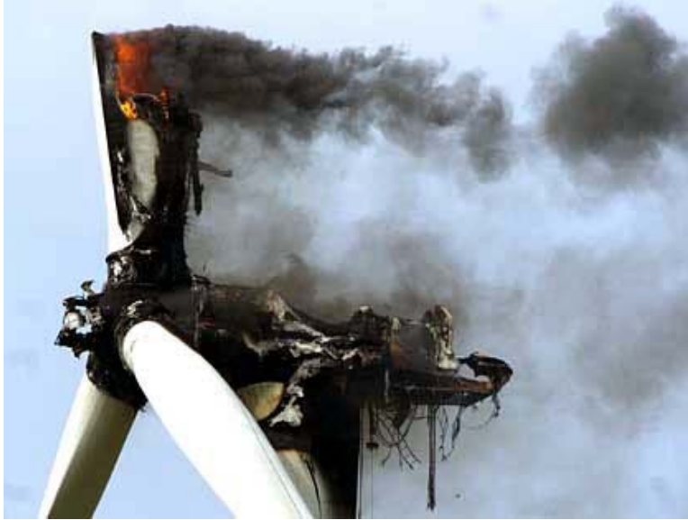
Figure 19. Fire caused by a short circuit, frictional overheating or lightning in 2004 in Germany. Source: Der Spiegel, DPA.
