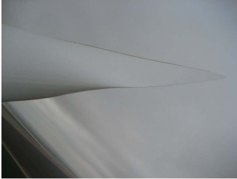
Figure 21. Structural crack caused by manufacturing defect in a rotor blade.
