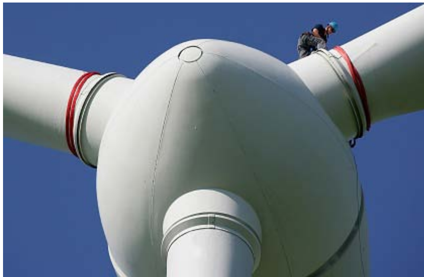
Figure 3. Assembly of wind turbine components entails work at great heights and use of safety harness equipment.
