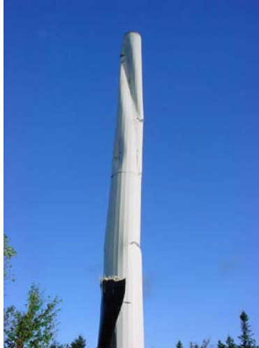
Figure 9. Turbine collapse in high wind conditions at the Searsburg, Vermont wind facility, September 15, 2008.
